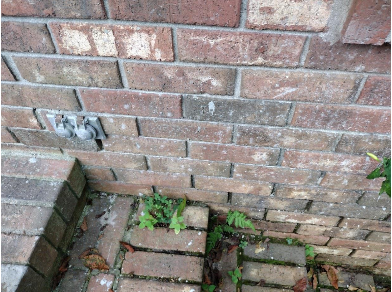
Thinset on brick porch, Photo 8. Thinset splattered onto brick siding.
