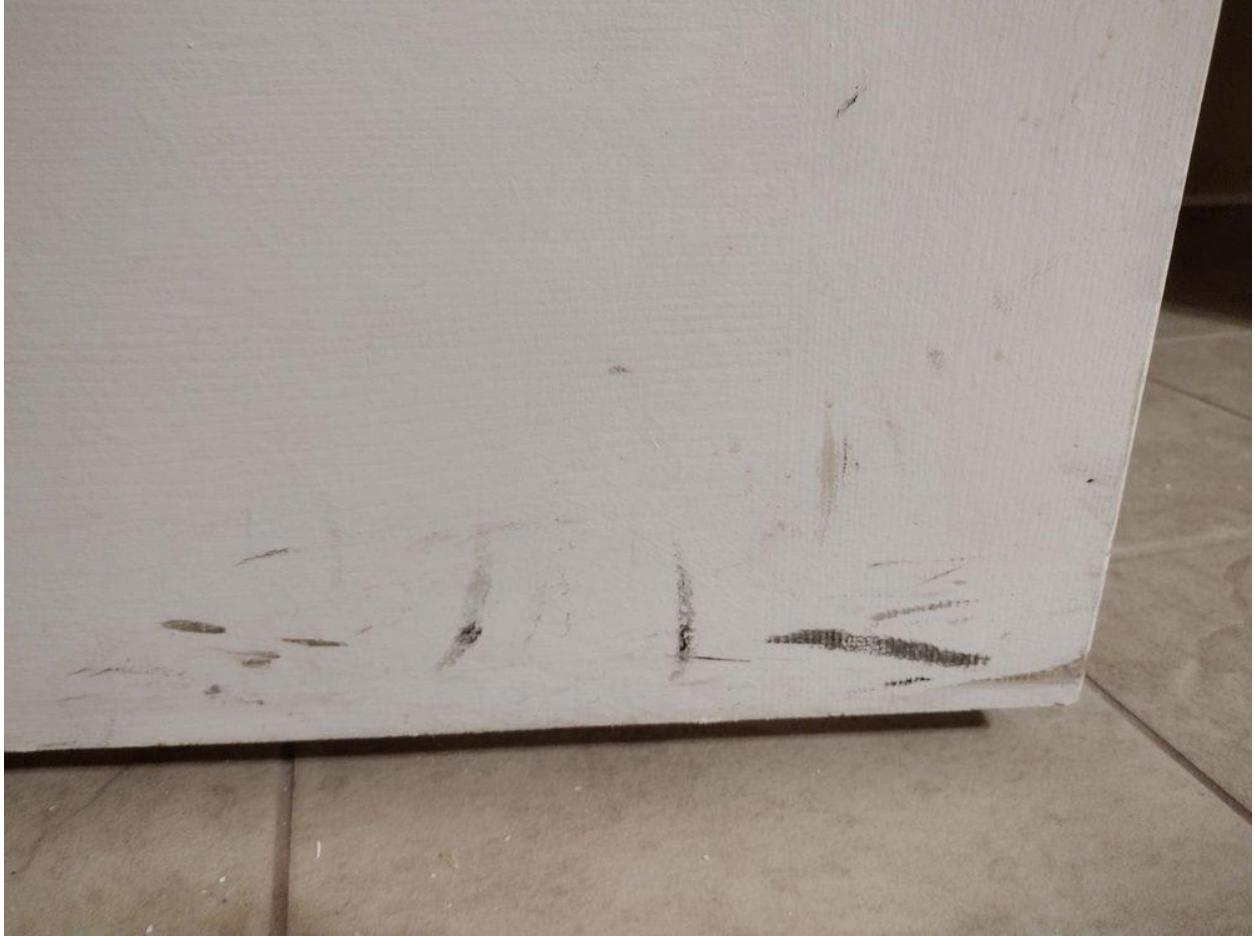
Grout on walls, Photo 4. Grout and thinset smeared on the doors.
