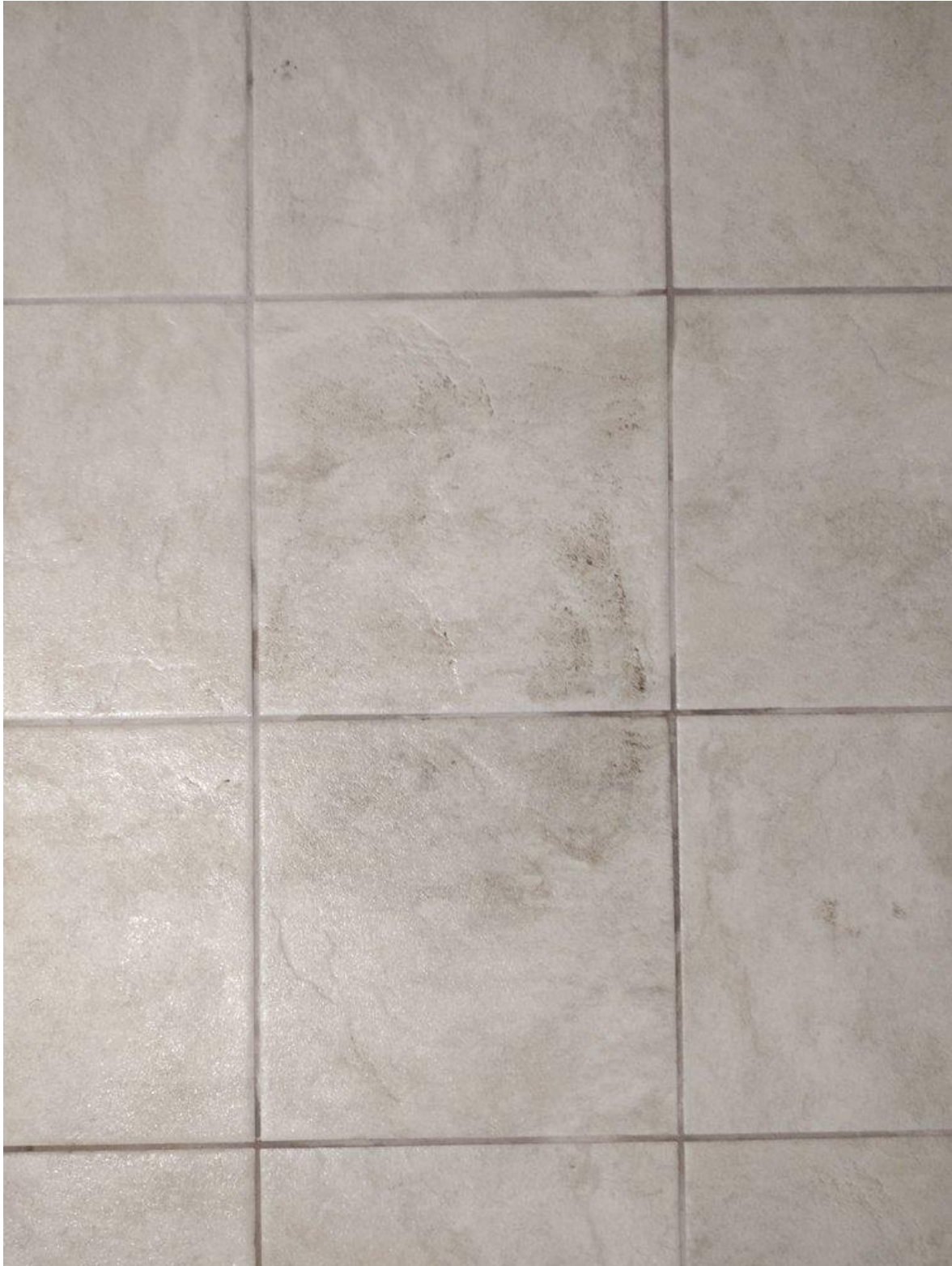
Grout cured on top of tiles, Photo 3. Grout cured on tile for a permanently dirty look.
