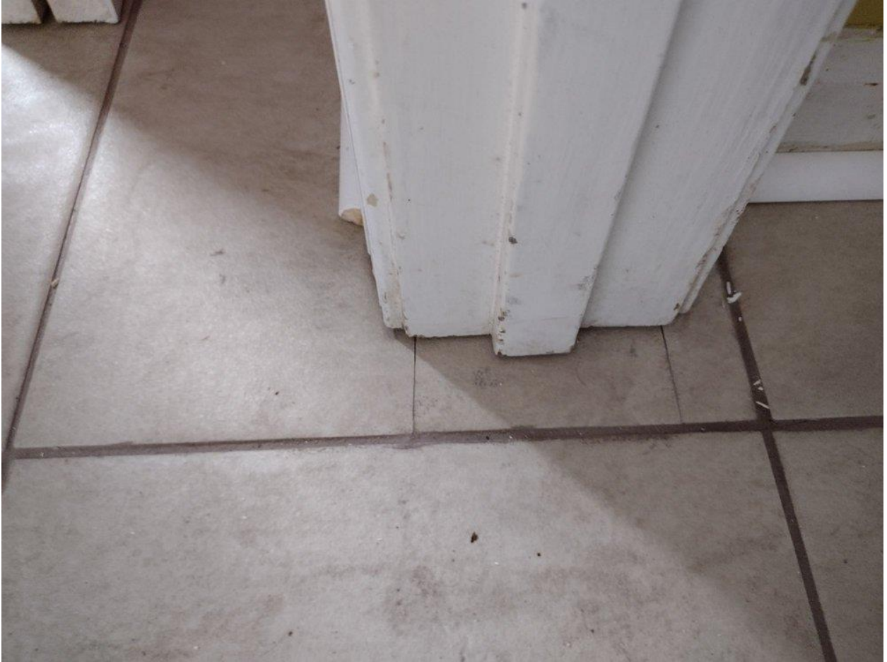
Tiles installed broken, Photo 2.
