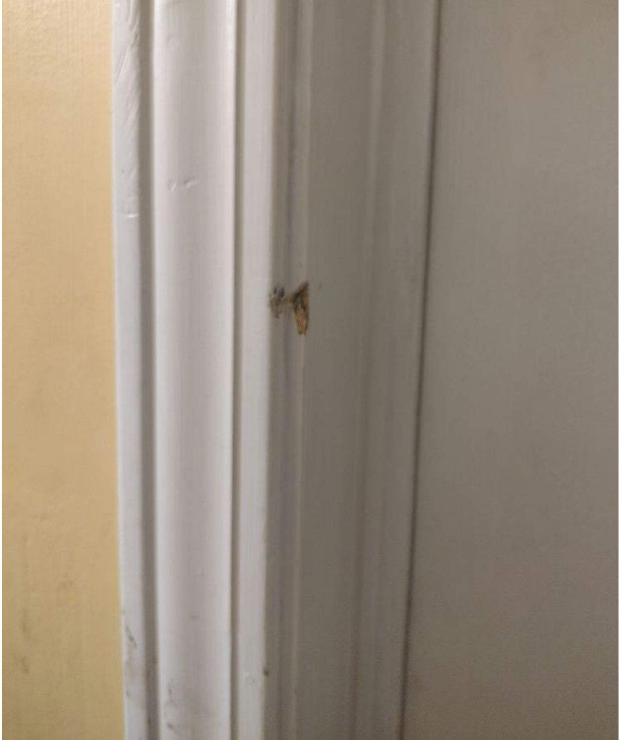
Grout on Walls, Photo 2. Chunk take out of door trim.
