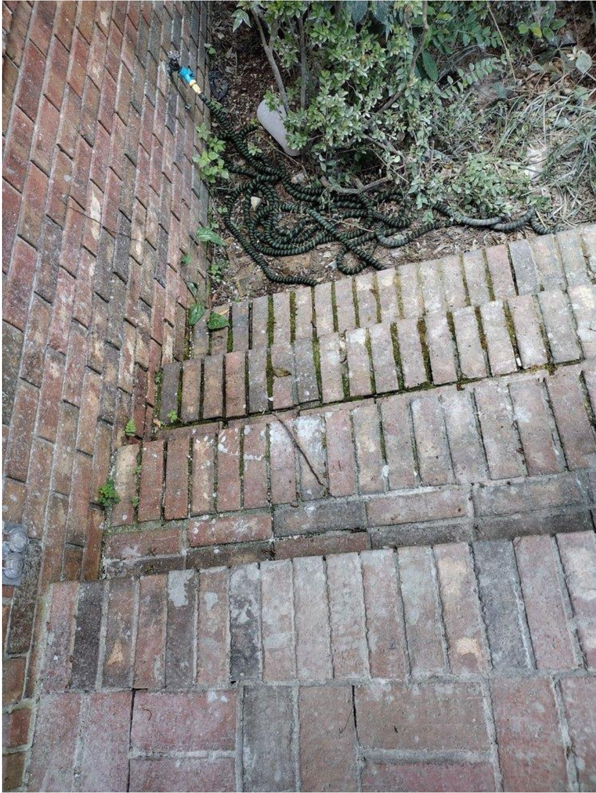
Thinset on brick porch, Photo 2. Thinset smeared on the brick porch.
