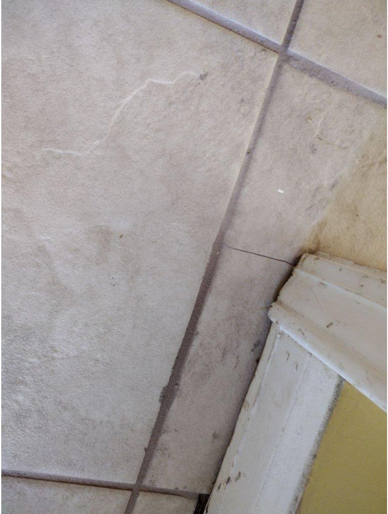
Tiles installed broken, Photo 3.
