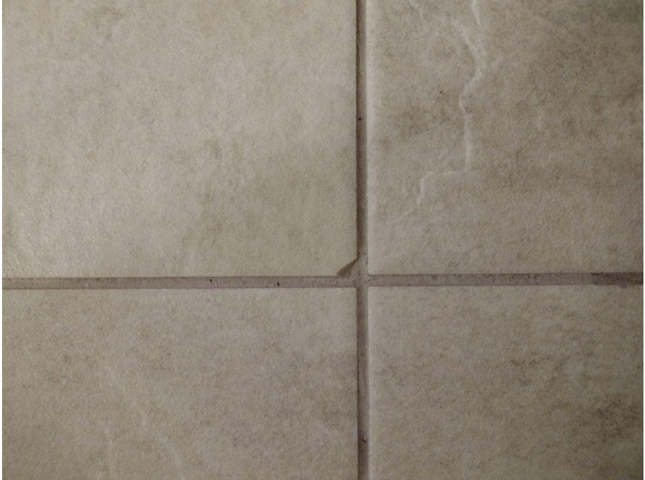
Tile installed chipped, Photo 1.
